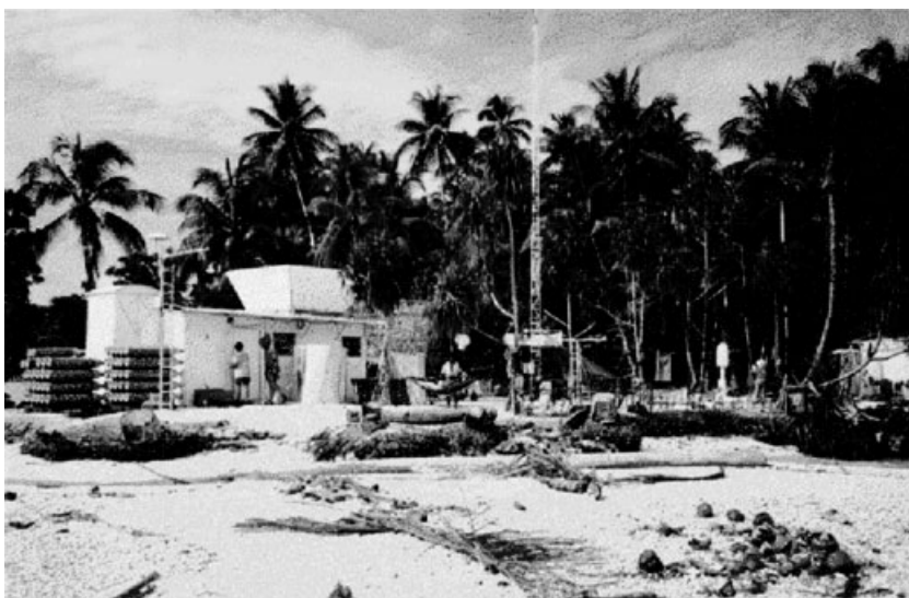
Figure 21 NCAR ISS in Kapingamarangi, Pohnpei State, Federated States of Micronesia. A wind profiler antenna is pointed vertically and shrouded by a clutter fence visible on top of the shelter. Aluminum cylinders shield a portion of a RASS radio acoustic sounding system. See ftp site for color image.
